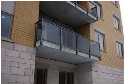
Photo 8: Balcony Offset Point Supports. Precast balcony supported intermittently to break thermal bridge.
