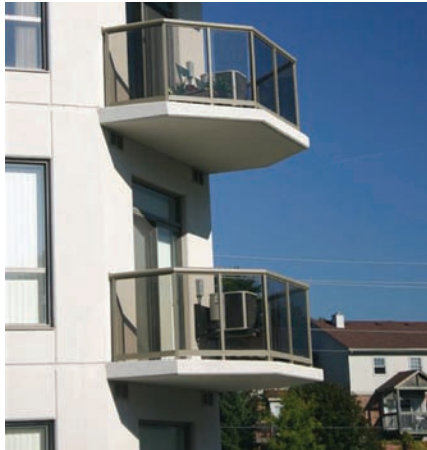
Photo 7: The Ultimate Thermal Bridge. A balcony is an efficient concrete-to-air heat exchanger that transfers every last available Btu across the structure.
