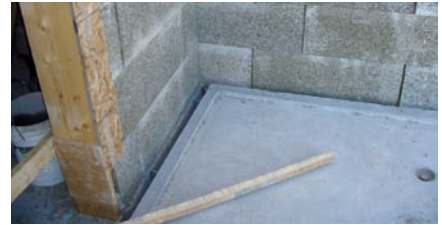
Photo 9: Mind the Gap. Closeup of precast balcony supported intermittently. Note the gap between the balcony and the structure allowing exterior insulation to run by.
