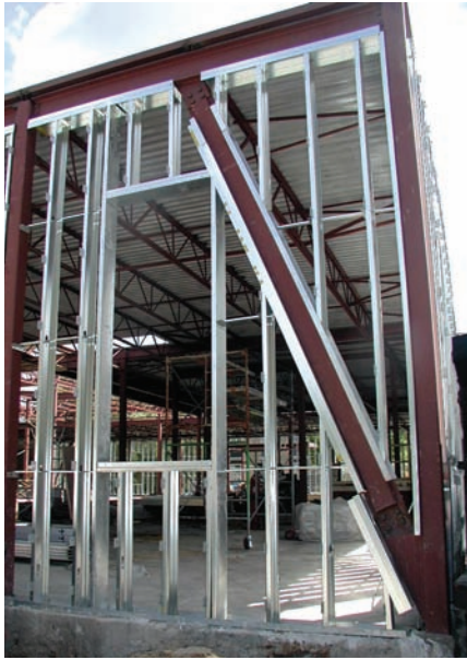
Photo 4: Conductive Heaven. Not much to say here except “what were you possibly thinking?” It is a waste to insulate the cavities. Exterior insulation is the only rational option here.
