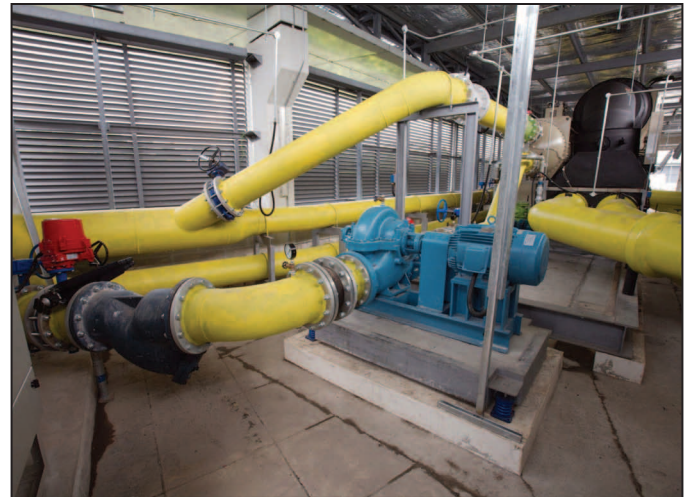
Figure 7: A Factor Ten design by Eng Lock Lee, with larger-diameter pipes and smooth transitions instead of right-angle bends.
