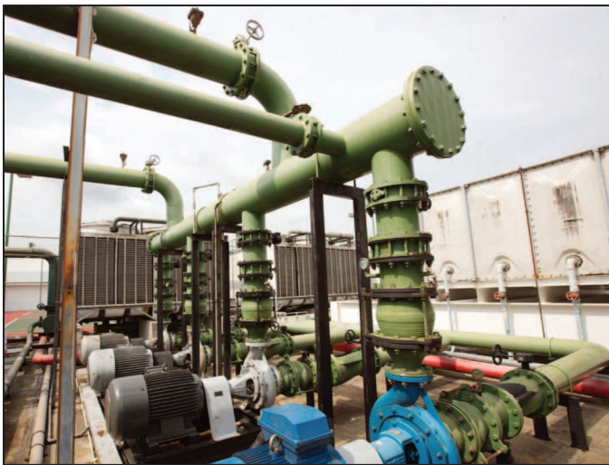
Figures 2 and 3: Typical piping layouts like these look pretty and are easy to draw. But the long pipes, right-angle bends and friction-adding control valves make the system less efficient.
