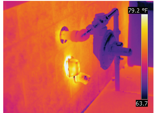
Figure F30. Infrared thermogram reveals air leakage at the electrical penetration while building was under pressurization.
