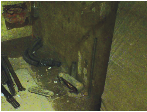
Figure F11. Derelict conduit penetration in concrete slab.
