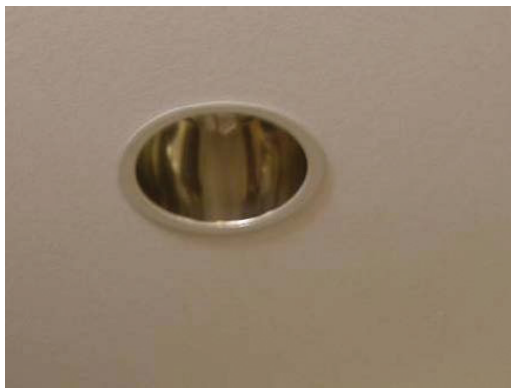
Figure F19. Recessed light penetrating the ceiling GWB that was intended to be the air barrier.
