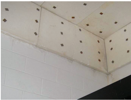
Figure F13. Insulation pinned to a below grade CMU wall
