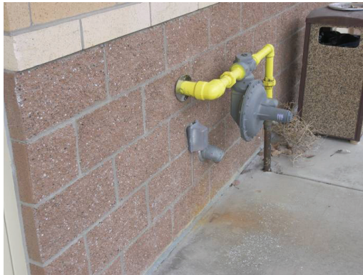
Figure F29. Electrical and gas utility penetrations in the enclosure
