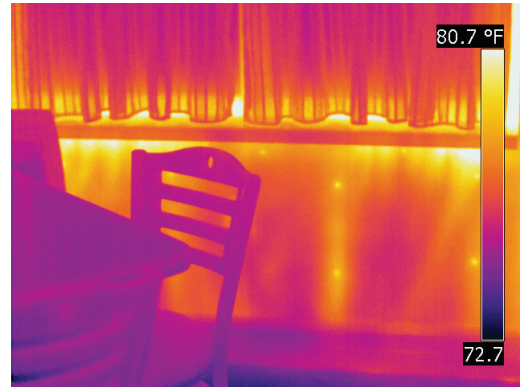
Figure F18. Infrared thermogram reveals air leakage at window sill while enclosure is depressurized.
