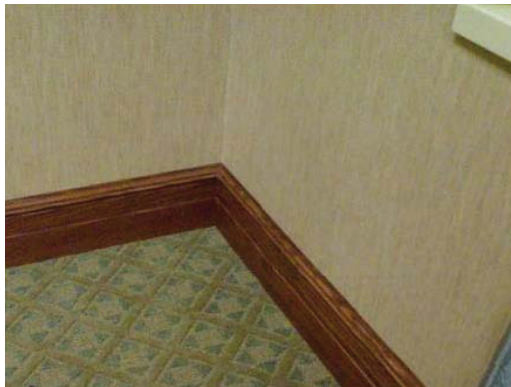
Figure F21. Base trim in a commercial facility with exterior wall on the right and interior wall across the top/left.
