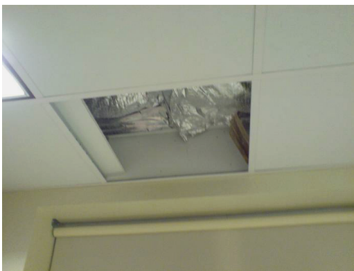
Figure F15. Removed drop-ceiling tile reveals foil faced insulation being used as the formal plane of building enclosure.
