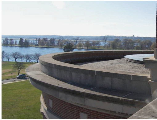
Figure F27. Roof detail on a historical renovation of a federal building
